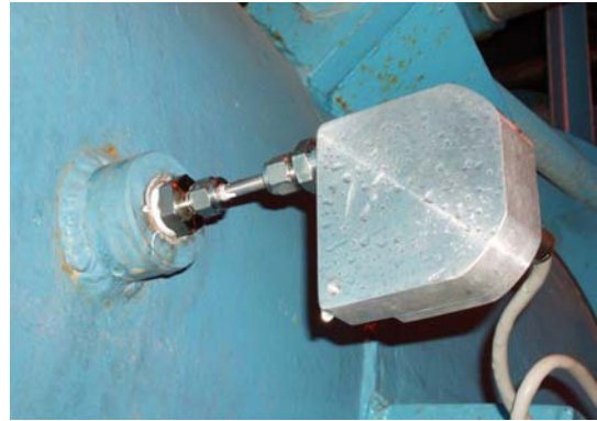
Figure 1: Fixed installation for continuous monitoring. The temperature probe is inserted into a thermowell.
