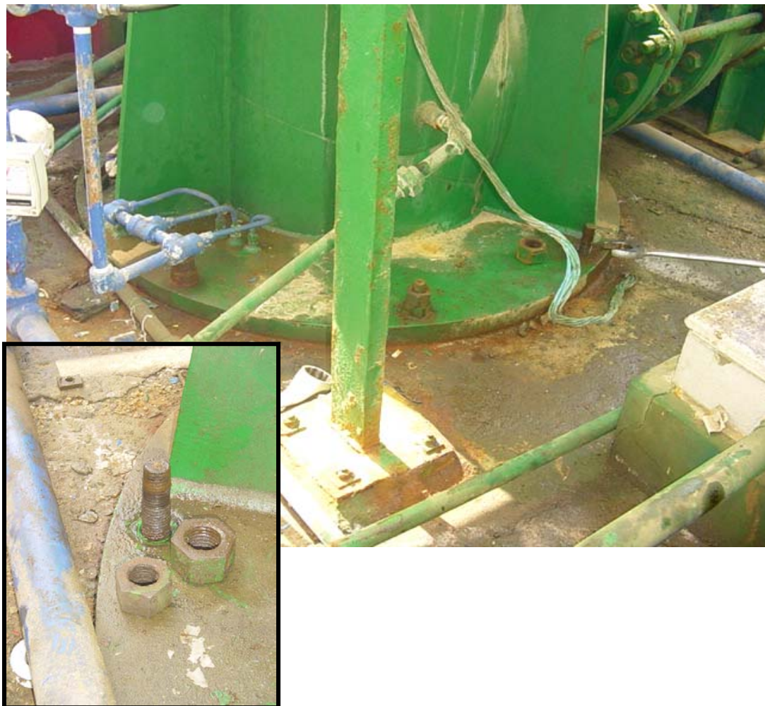
Figure 6 Physical deterioration in the foundation, bolts and nuts
